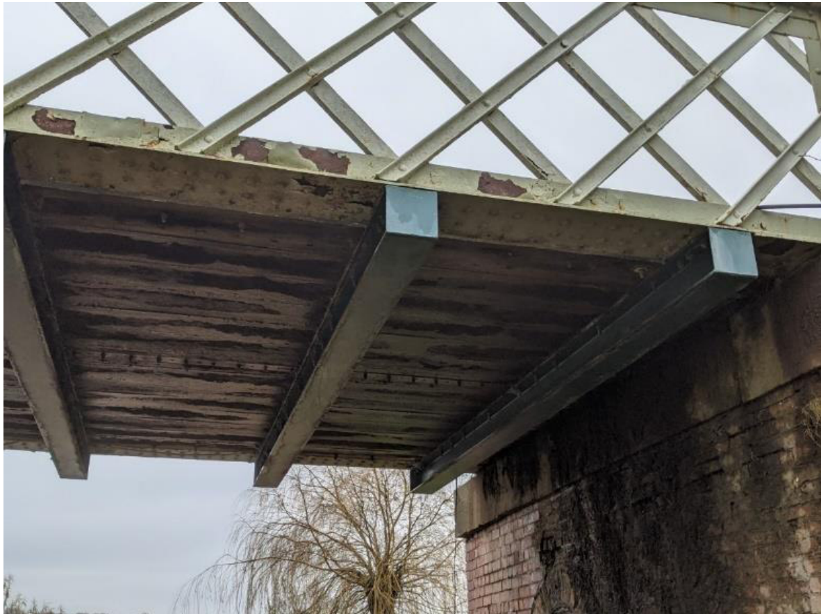
Figure 4: The two main horizontal beams spanning the river are interconnected with cross beams underneath, now replaced with new sections in steel.
