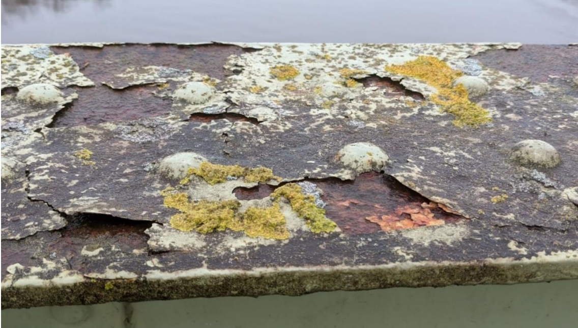
Figure 11: Close up of the damaged coating at the top surface of the parapet with corrosion taking place underneath the protective coating and lichen growth being encouraged.
