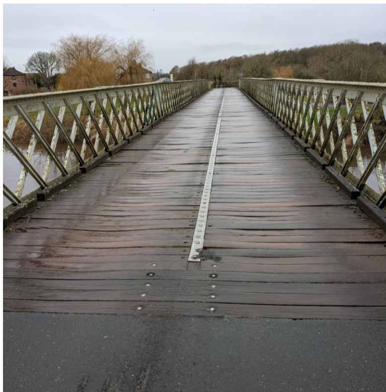
Figure 14: The top decking as viewed from the east approach. The uneven surface is evident with boards having sunk and others projecting.
