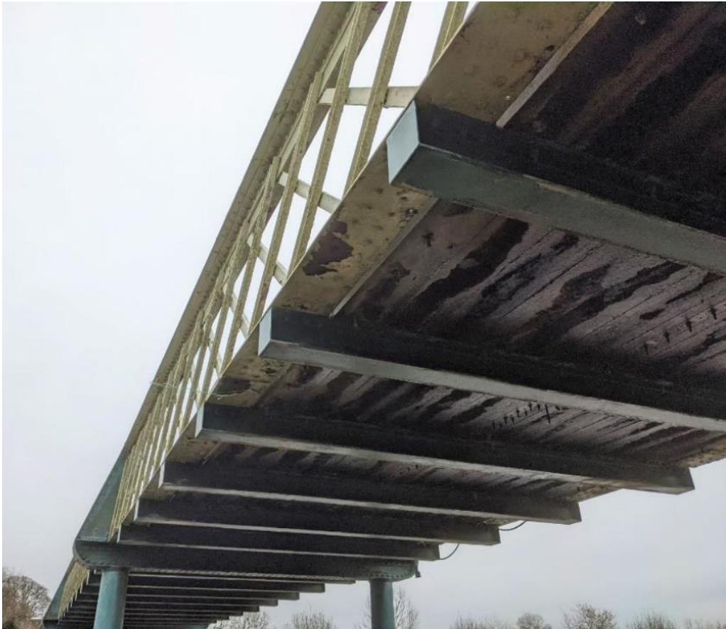
Figure 7: A bottom layer of timber boards is fixed across the crossbeam spans. A steel strap fixed along them is evident in the middle of the bridge width.
