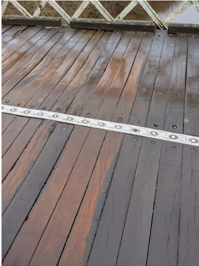
Figure 5: The top decking is demarcated by a double row of bolts holding down the inner ends of the boards, the one row further aligned with a steel strap.
