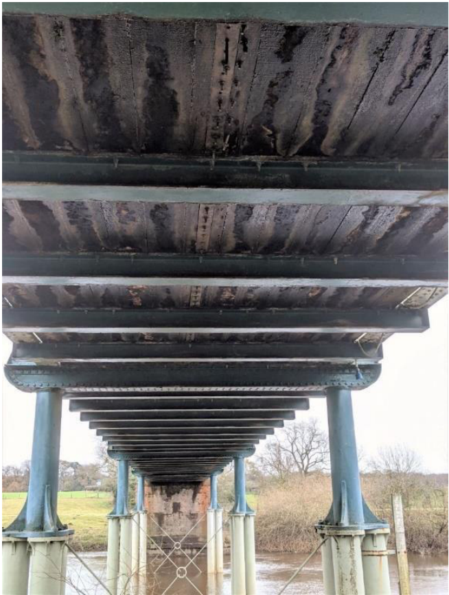
Figure 18: The bottom layer of the decking is extensively stained due to the general wet conditions and the inadequate drainage.
