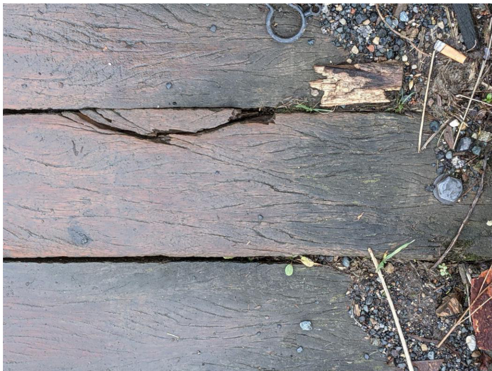
Figure 15: Timber boards with broken pieces and debris around, encouraaina veetation growth..
