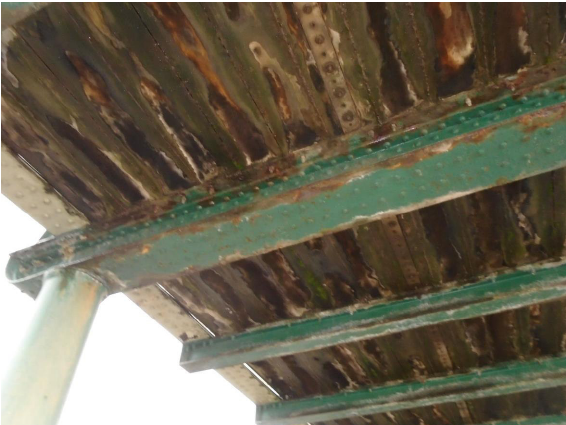
Figure 12: Corrosion has taken place to a significant degree to the cross beams below the timber decking.
