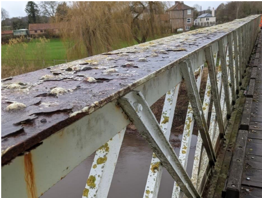
Figure 10: Protective coatings to metalwork are damaged and flaking leaving the metal surface vulnerable to corrosion. This is particularly evident at the top surfaces of the parapets.
