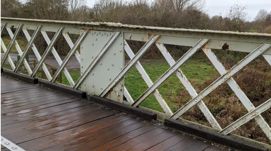
Figure 13: Deterioration extends to more protected elements which are stained with dirt and lichen growth, which will eventually affect the coating which will deteriorate further.
