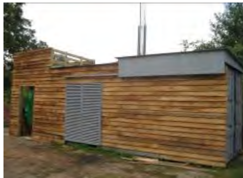
Oak clad woodfuel boiler
