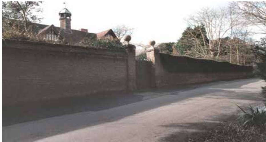
Figure 5.56 The Garden Wall and Gateways to North of Milstead Manor as viewed from Manor Road
