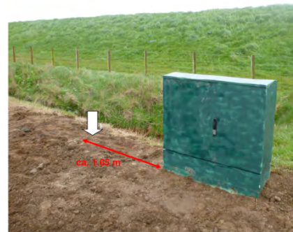
Figure 4.6: Indicative illustration of Traffic light monitoring equipment
